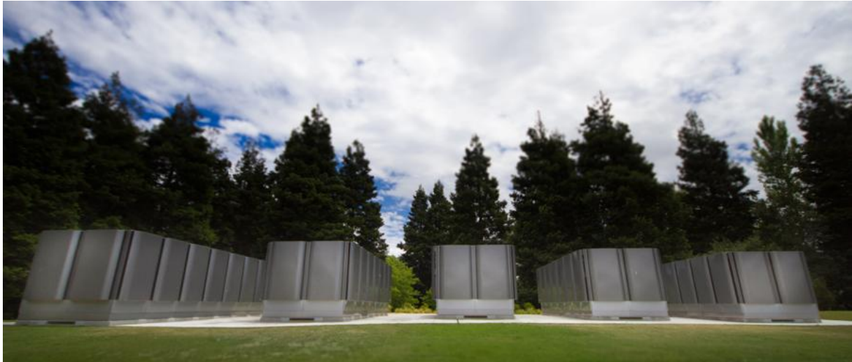
A Bloom Energy fuel cell installation in the USA (Source: Bloom Energy)
